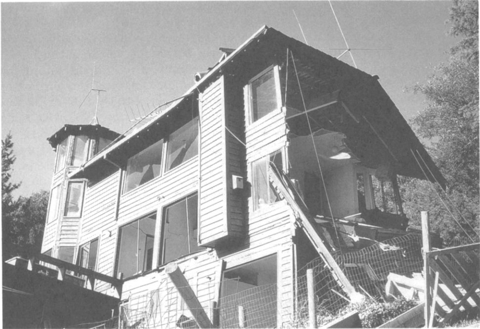
FIG. 2. The facade of the home pictured here, high in the Santa Cruz Mountains, looked south across Monterey Bay to the Monterey Peninsula beyond. Failure of this structure occurred in several ways, the result of strong ground motion, possibly topographically amplified, and slope failure. The deck in the lower left of the picture was formerly attached to the house at the first floor level beneath the sliding glass doors just to the left of the chimney well.
